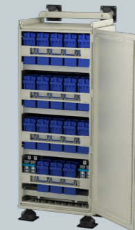
CENTRAL SYSTEM BATTERY CABINET
